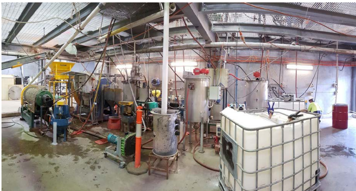
Figure 1: Flotation Pilot Plant – Milling, Conditioning, De-slimes and Reagents
